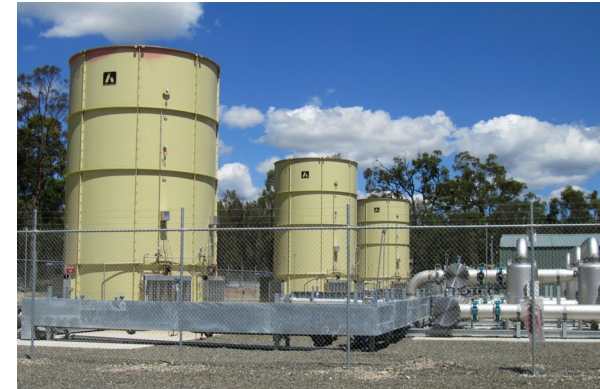
Drainage gas flaring facility at a mine (2016)
