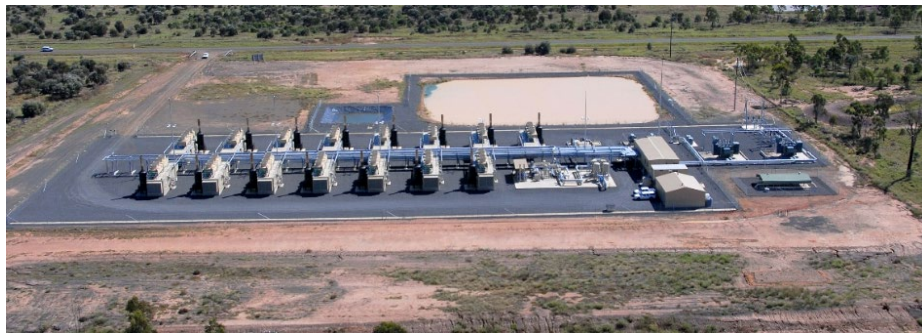
A 63MW Power Station utilising coal mine gas (Source: Clarke energy)
